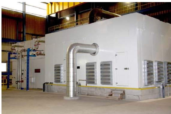
Essar Power Co-Generation Facility
